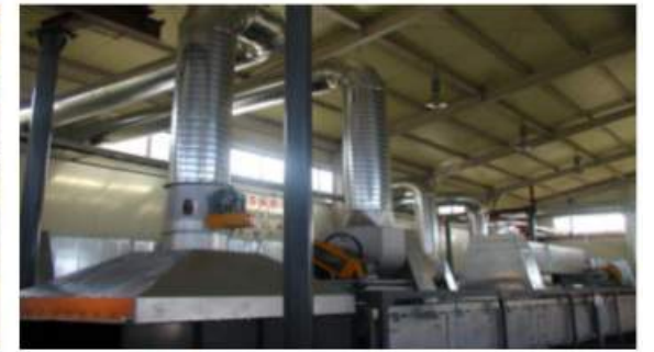
건조 Line (Booth & Duct)
